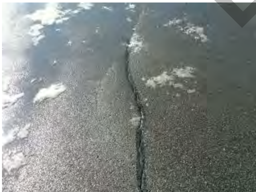
Cracking At Asphalt Joint
