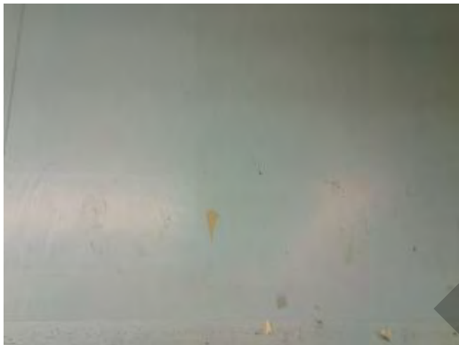
Chipped And Faded Interior Walls
