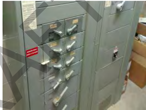
Main Distribution Panel
