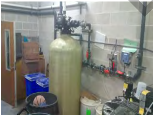
PH Controls & Tank
