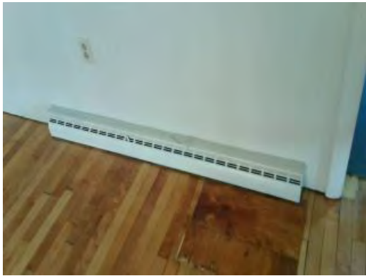
Damaged Baseboard Heater
