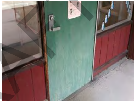
Faded Exterior Door
