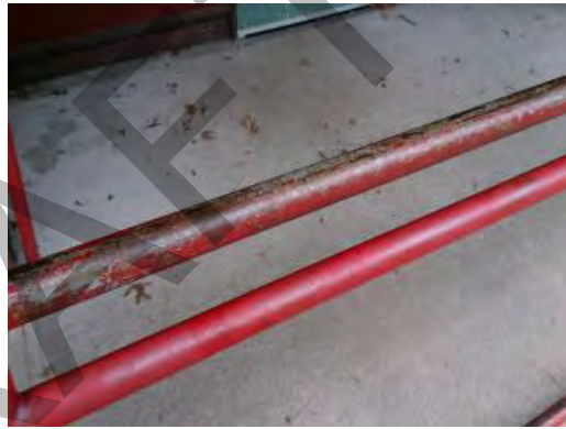
Typical Worn Handrail
