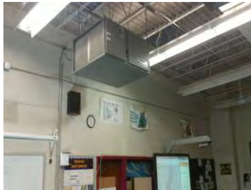
Main Building - Poorly Functioning Unit Heater
