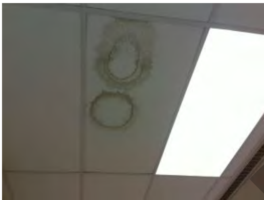
Stained Ceiling Tile
