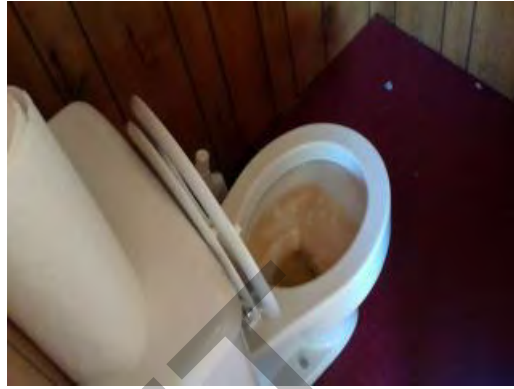
Aged And Stained Toilet
