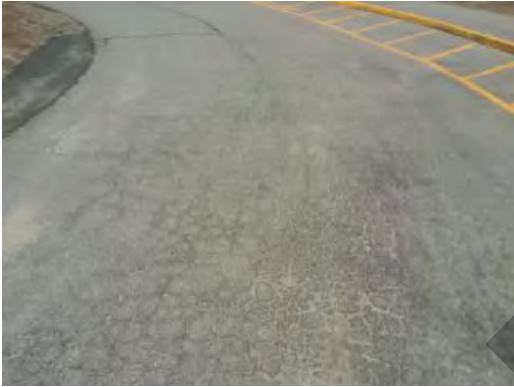
Cracking Asphalt Paving
