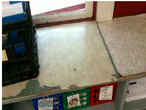
Chipped And Worn Cabinetry
