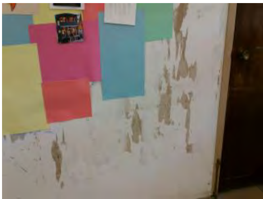
Main Building - Damaged Painted Classroom Wall
