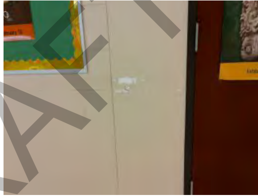
Typical Chipped Paint
