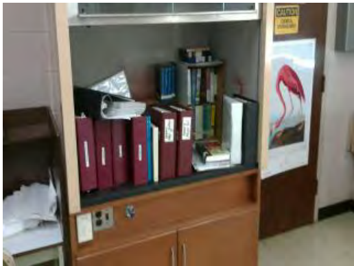
Main Building - Inoperable Fume Hood Used As Storage
