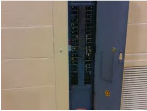
Main Building - Typical Aged Panelboard
