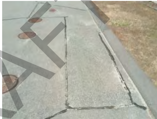
Damaged Play Area Asphalt
