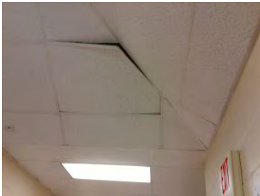
Ceiling Tile Falling Out Of Grid
