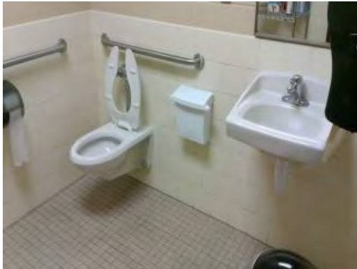
Staff Restroom Fixtures And Finishes
