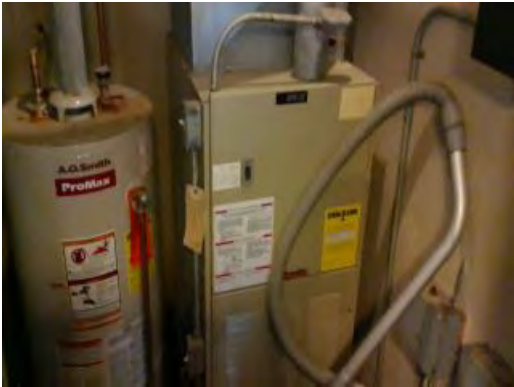
Furnace And Water Heater
