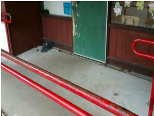
Chipped And Faded Exterior Door
