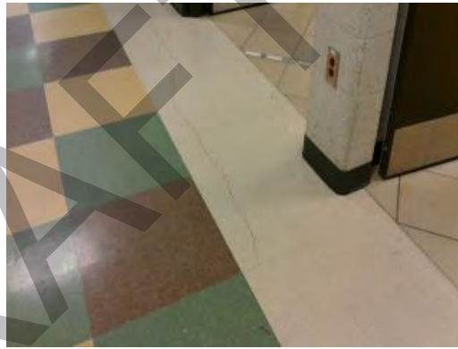
Cracked VCT Floor
