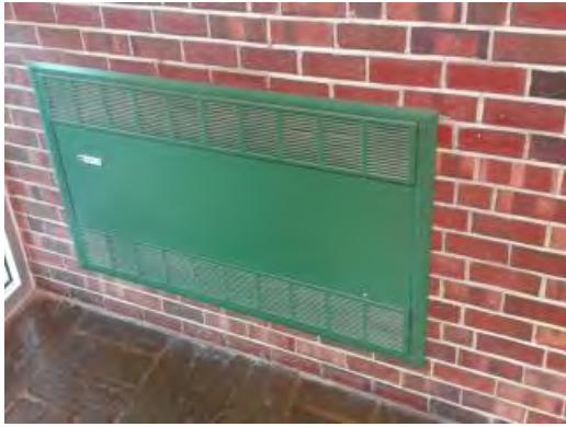
Main Building - Original Hallway Unit Heater
