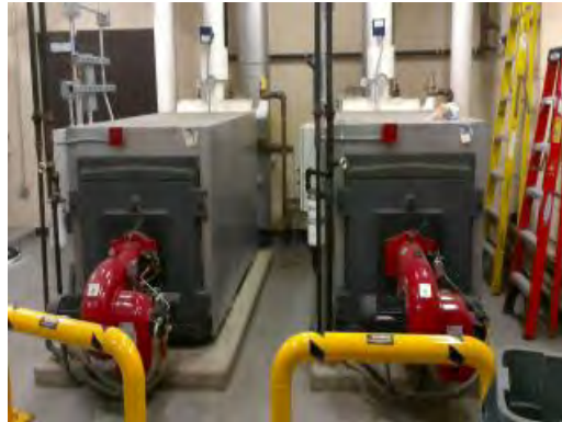
Heating Water Boilers
