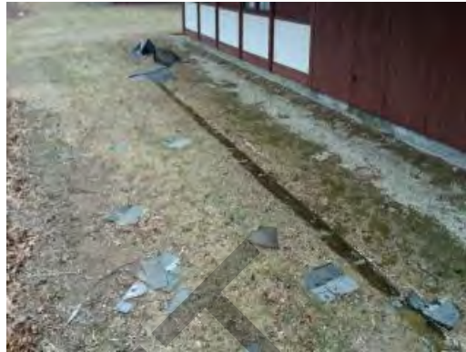
Displaced Roof Shingles
