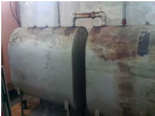
Fuel Oil Storage Tanks
