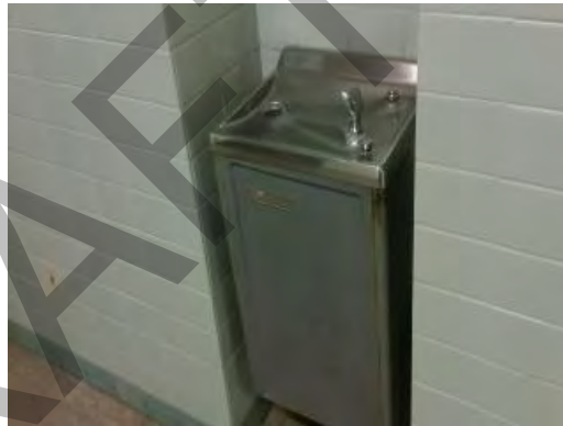
Main Building - Non-Functional Drinking Fountain
