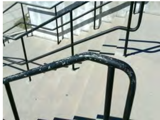
Main Building - Chipped Paint On Handrail
