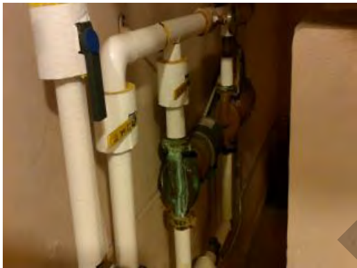
Main Building - Abandoned Circulators
