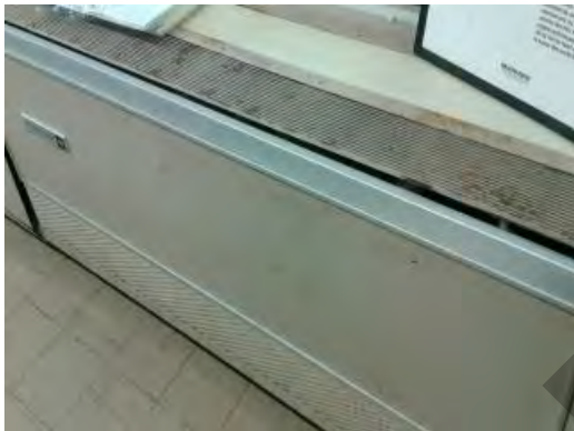
Main Building - Aged Heating Unit Ventilator
