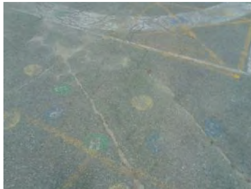
Cracked, Worn Play Area Asphalt
