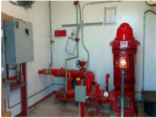
Fire Pump House - Interior
