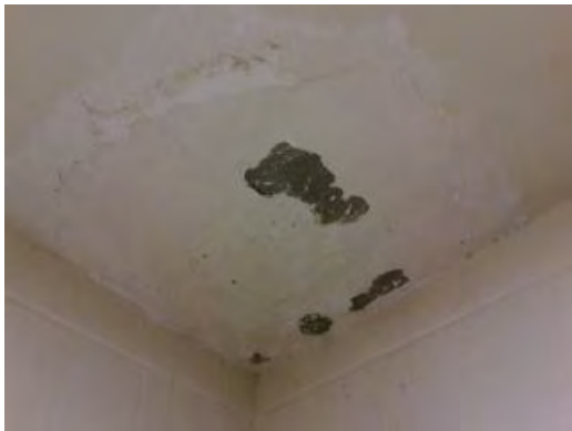
Main Building - Paint Peeling And Bubbling On Ceiling
