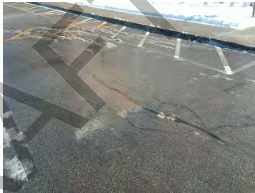
Cracking Asphalt At Main Drain
