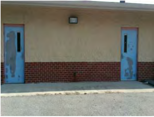
Typical Worn Metal Exterior Doors
