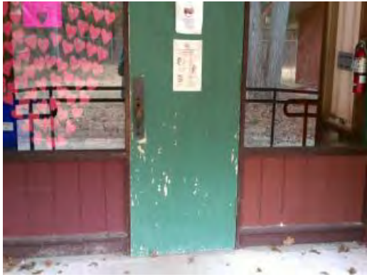
Chipped And Faded Exterior Door
