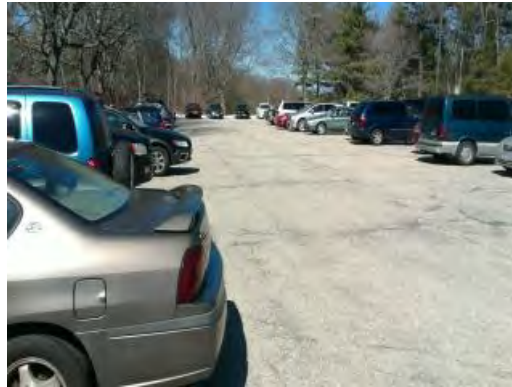
Site - Cracked And Worn Asphalt Parking Lot
