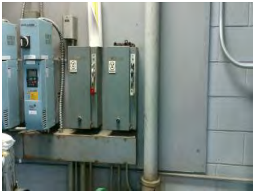
Main Building - Abandoned Electrical Disconnects
