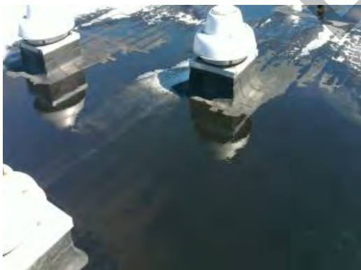
Main Building - Typical Exhaust Fans
