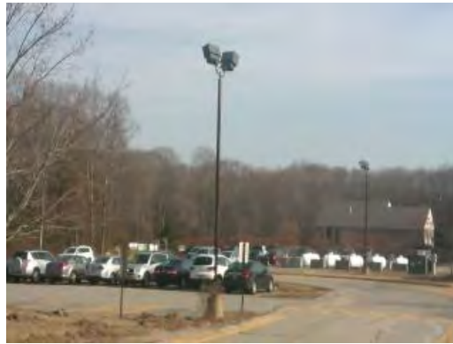
Rusted Pole Mounted Lights
