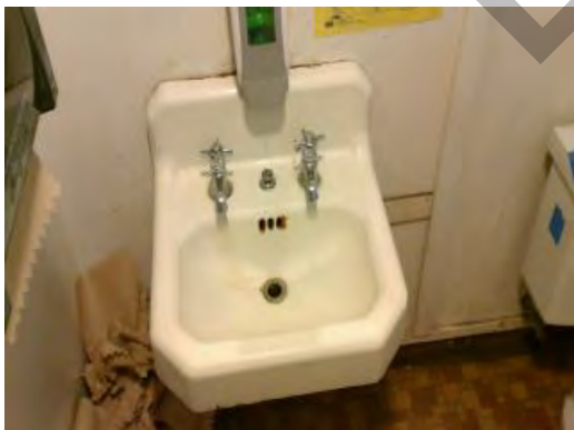
Typical Lavatory Fixture
