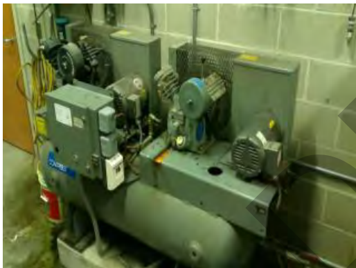
Pneumatics System Leaking
