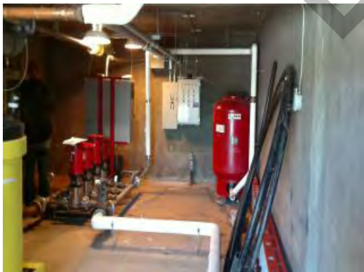
Pump House - Interior
