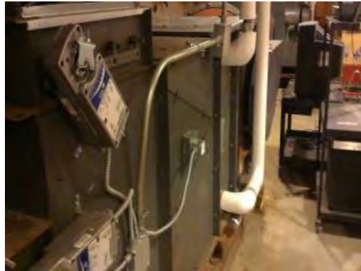
Main Building - Original AHU
