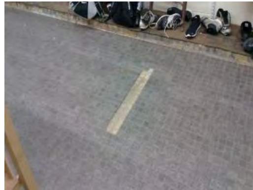
Main Building - Missing Ceramic Tiles
