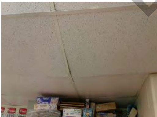
Bent Ceiling Grid
