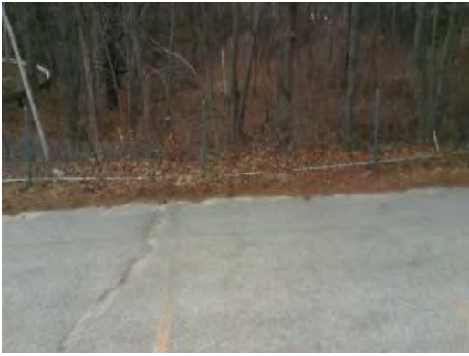
Fence Falling Down
