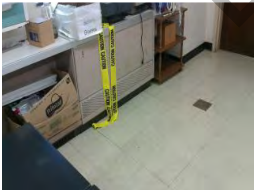
Main Building - Failed Classroom Unit Heater
