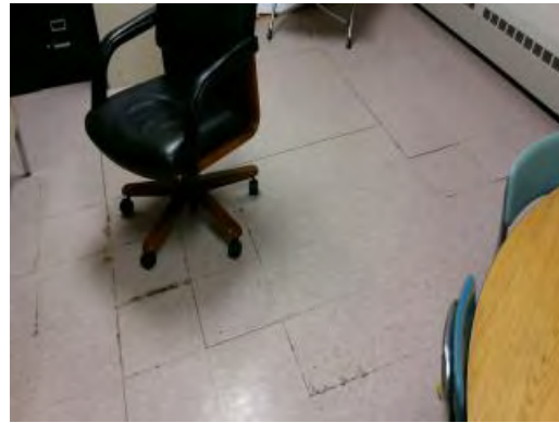
Typical Worn VCT
