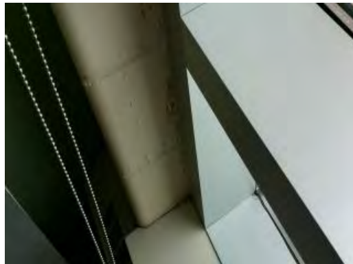
Failed Sealant Allowing Leaks
