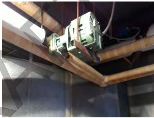
Main Building - Original Pump
