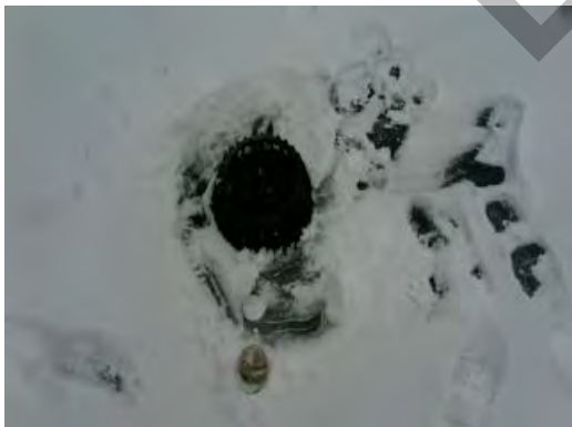
Blocked Roof Drain
