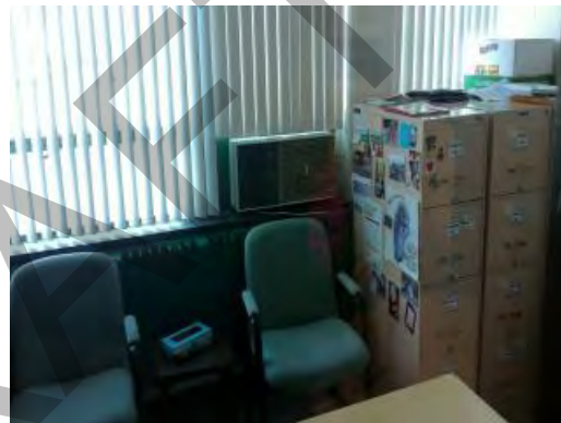
Main Building - Non-Functional Window Unit
