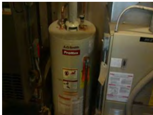
Rusted Water Heater
