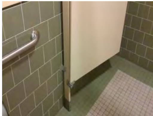
Crooked Toilet Partition
