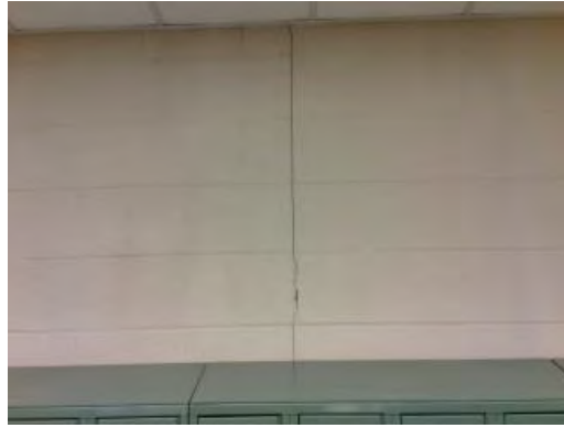
Cracked CMU Wall
