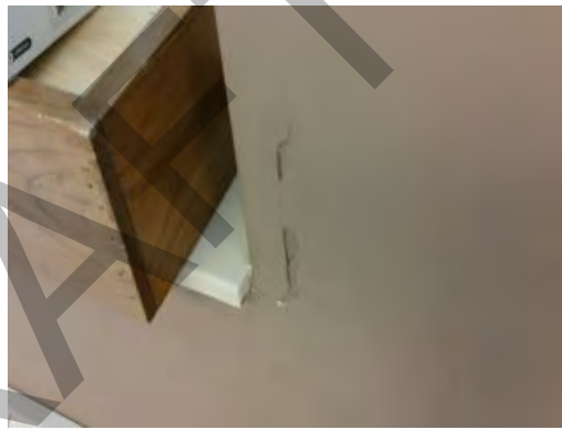
Damaged Gypsum Board Wall
