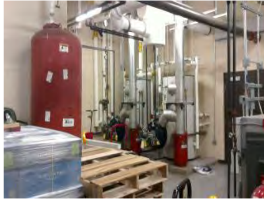
Domestic Water Boilers
