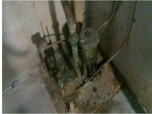
Main Building - Inoperable Sump Pump
