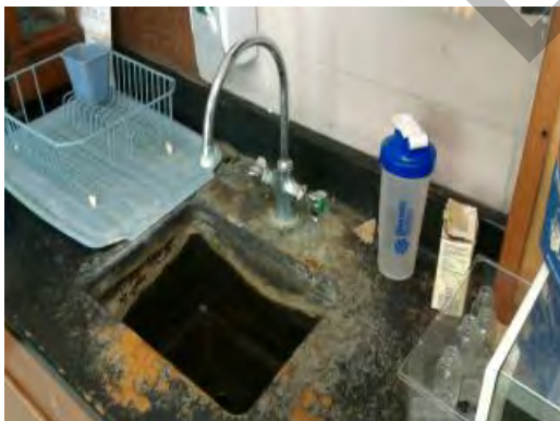
Main Building - Corroded Classroom Sink
