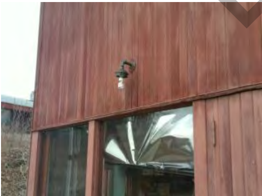
Building Mounted Light
