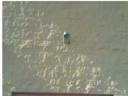
Broken Building Mounted Light
