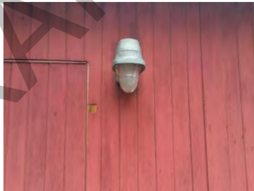
Building Mounted Light
