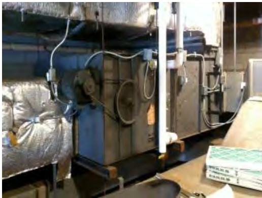
Main Building - Original AHU
