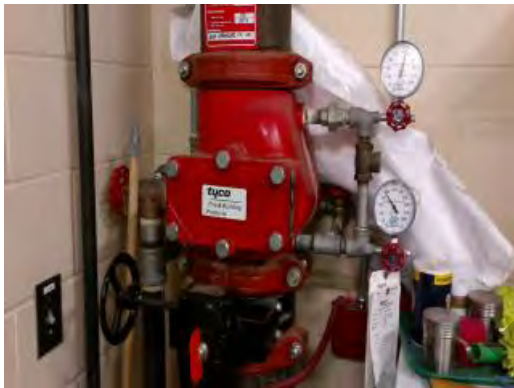
Fire Protection Entrance
