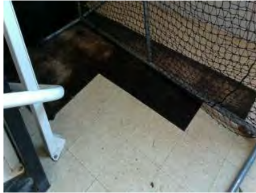
Main Building - Cracked And Missing VCT
