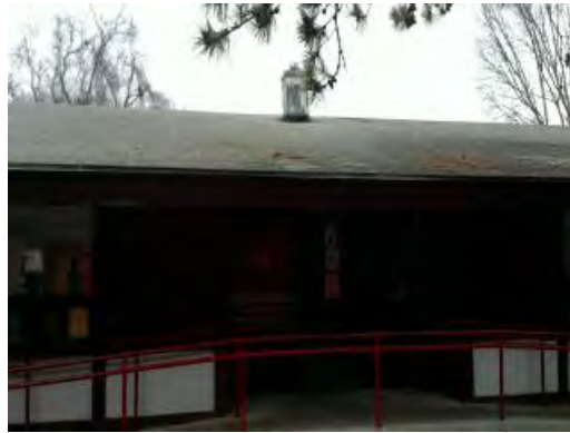
Shingles Missing From Building 2 Roof
