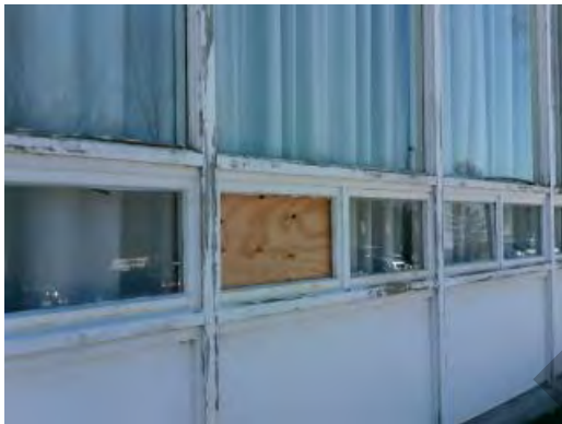
Main Building - Windows With Missing Pane
