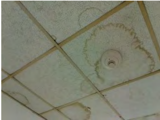
Main Building - Stained Ceiling Grid And Tiles
