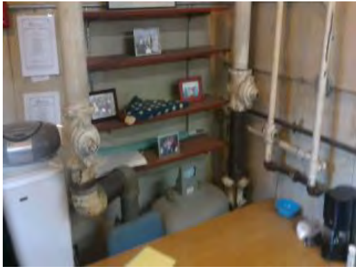
Gas Service Valve
