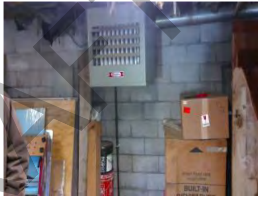
Maintenance Shed - Non-Functional Unit Heater
