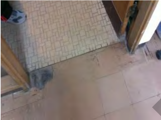
Typical Worn VCT
