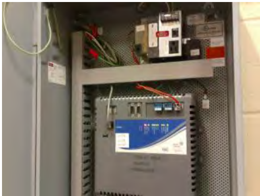
DDC Control Panel
