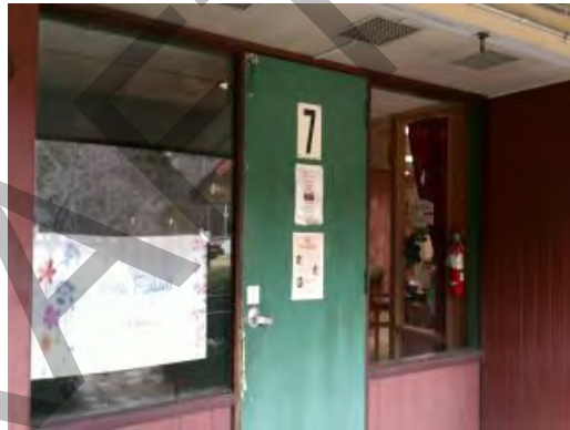
Faded Exterior Door
