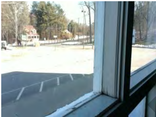
Main Building - Cracking Wood Framed Window
