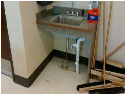
Pipe Missing Insulation
