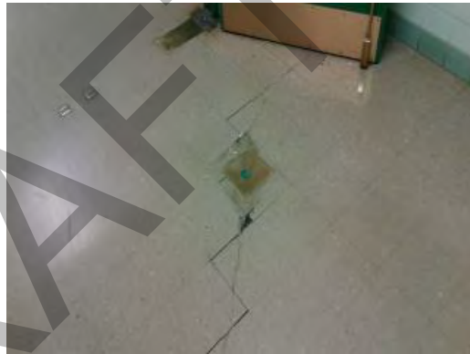
Main Building - Cracked And Separating 9x9 Tile
