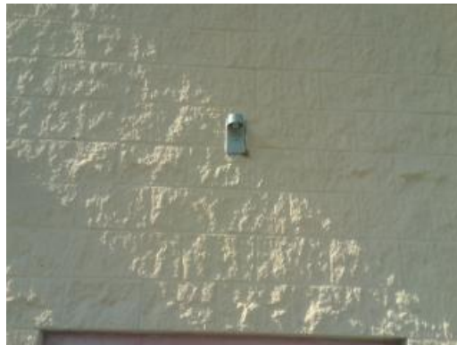
Broken Building Mounted Light
