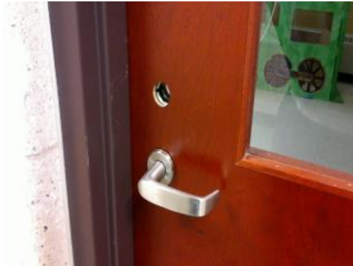
Missing Door Lock
