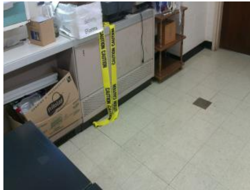
Main Building - Failed Classroom Unit Heater
