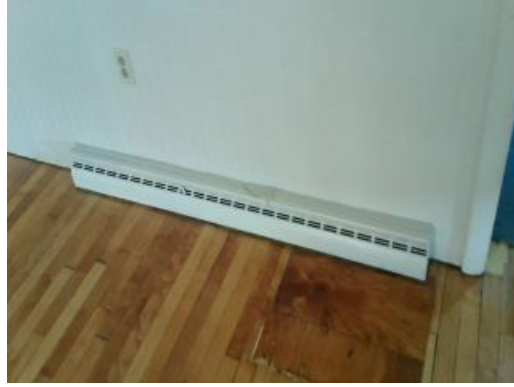
Damaged Baseboard Heater
