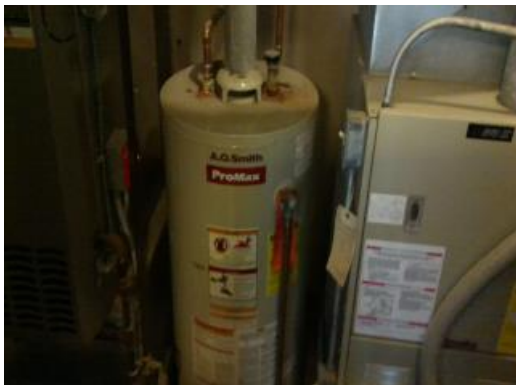
Rusted Water Heater
