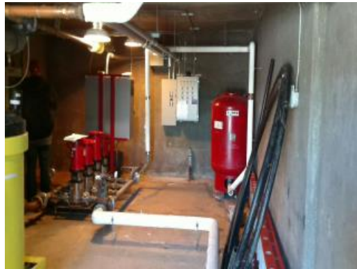
Pump House - Interior
