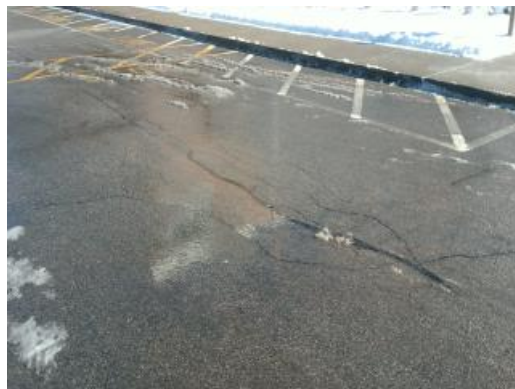
Cracking Asphalt At Main Drain
