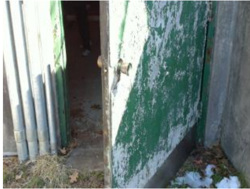
Pump House - Weathered Exterior Door
