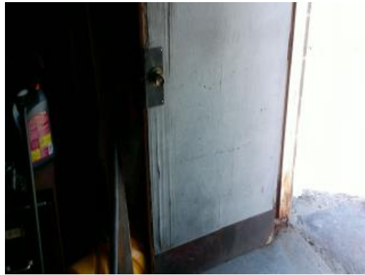
Maintenance Shed - Damaged Exterior Door
