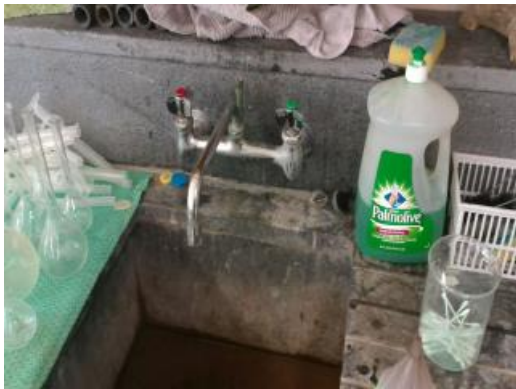
Main Building - Corroded Classroom Sink
