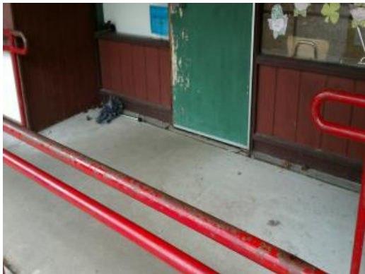
Chipped And Faded Exterior Door
