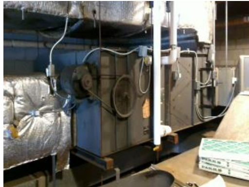
Main Building - Original AHU
