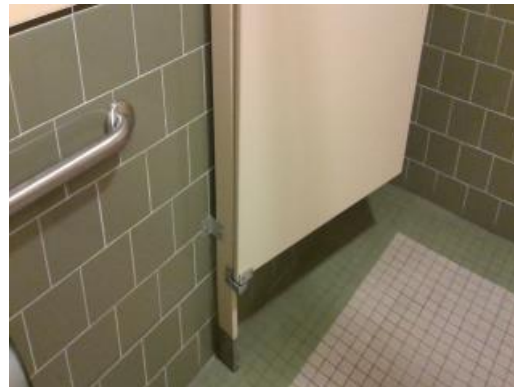
Crooked Toilet Partition
