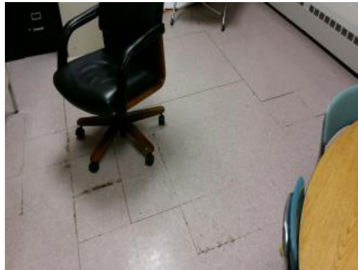
Typical Worn VCT
