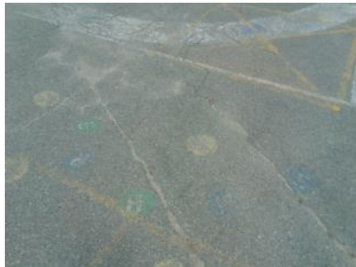
Cracked, Worn Play Area Asphalt
