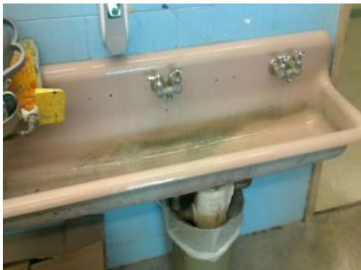
Main Building - Stained And Leaking Trough Sink Fixture
