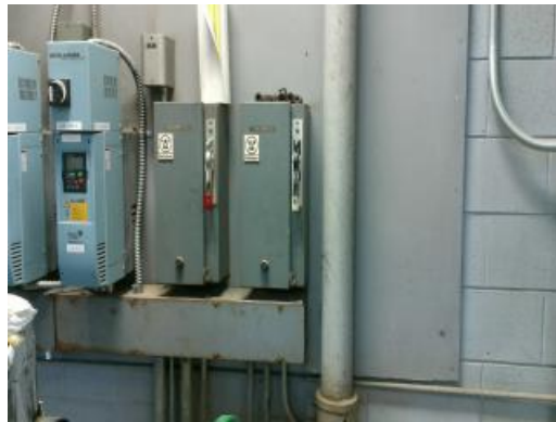
Main Building - Abandoned Electrical Disconnects
