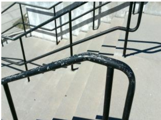
Main Building - Chipped Paint On Handrail
