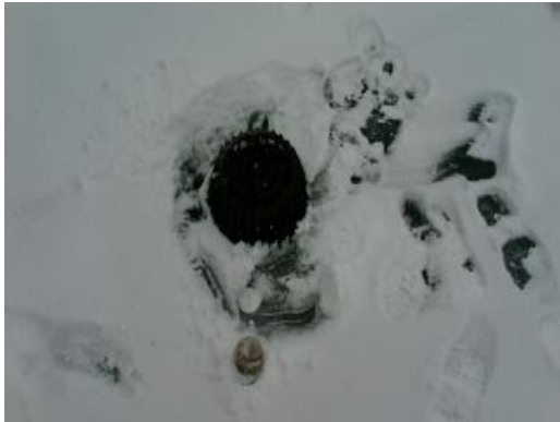
Blocked Roof Drain
