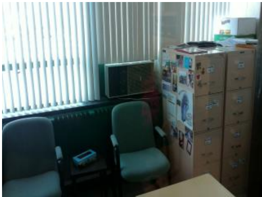
Main Building - Non-Functional Window Unit
