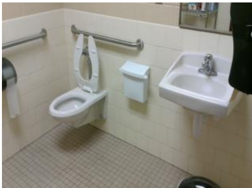
Staff Restroom Fixtures And Finishes
