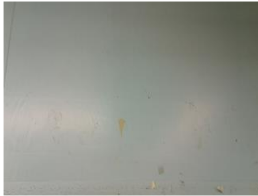
Chipped And Faded Interior Walls
