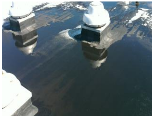
Main Building - Typical Exhaust Fans
