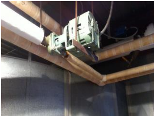
Main Building - Original Pump
