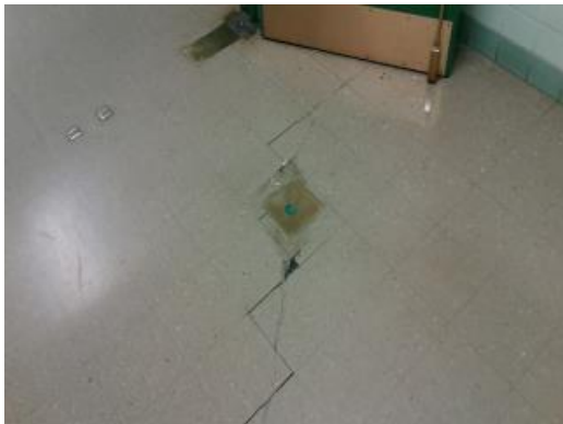
Main Building - Cracked And Separating 9x9 Tile
