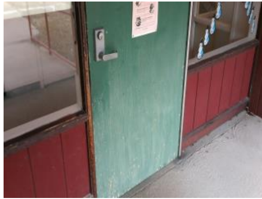
Faded Exterior Door
