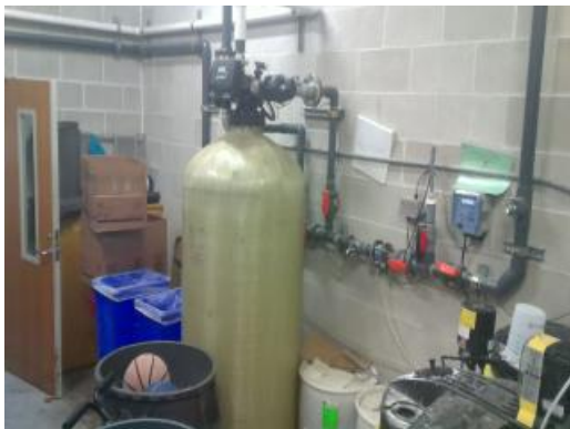
PH Controls & Tank
