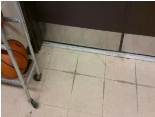
Worn And Stained VCT
