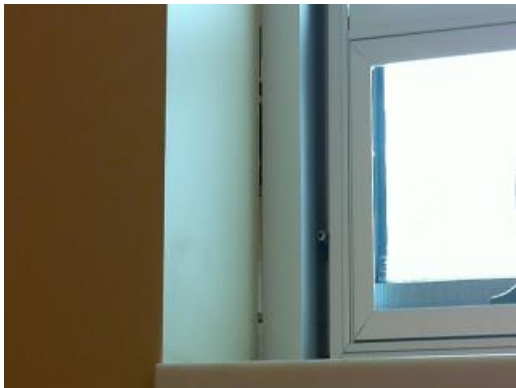
Sealant Failing At Window
