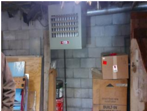
Maintenance Shed - Non-Functional Unit Heater
