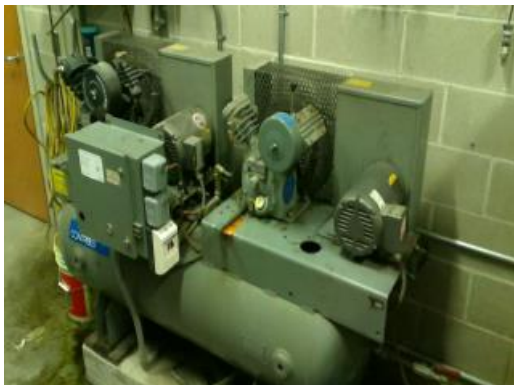
Pneumatics System Leaking
