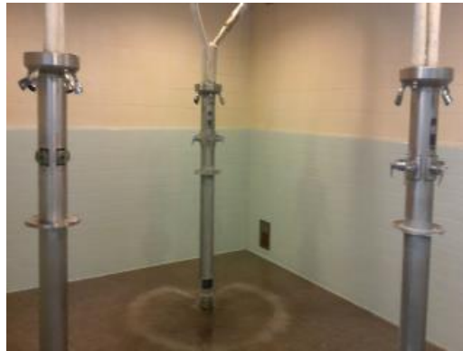
Main Building - Failing Shower Fixtures
