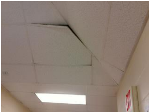
Ceiling Tile Falling Out Of Grid
