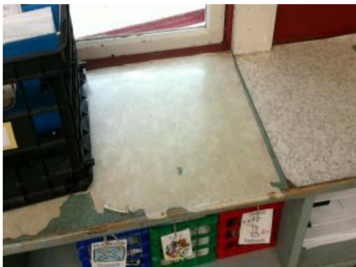
Chipped And Worn Cabinetry
