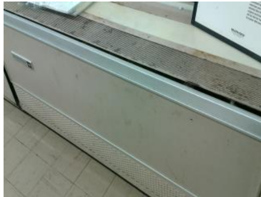
Main Building - Aged Heating Unit Ventilator
