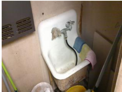
Stained Service Sink
