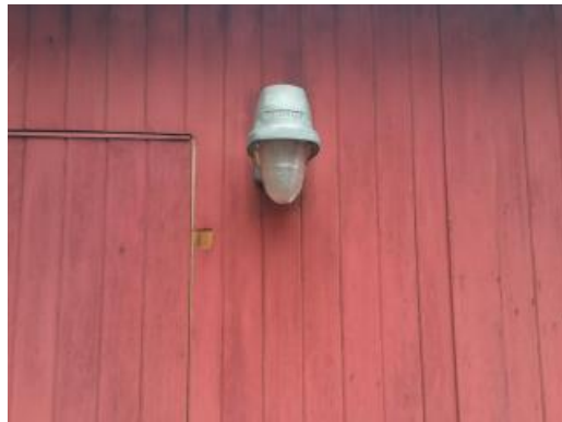
Building Mounted Light
