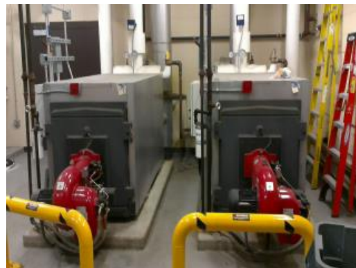
Heating Water Boilers
