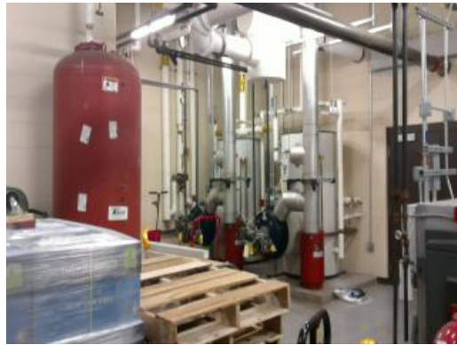
Domestic Water Boilers
