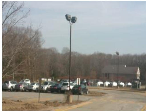
Rusted Pole Mounted Lights
