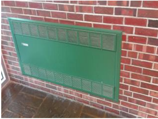
Main Building - Original Hallway Unit Heater
