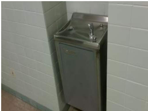
Main Building - Non-Functional Drinking Fountain
