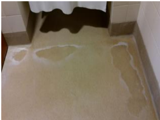
Water Damage Due To Floor Slope At Shower
