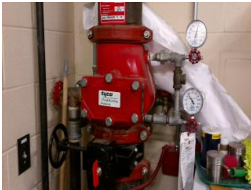
Fire Protection Entrance
