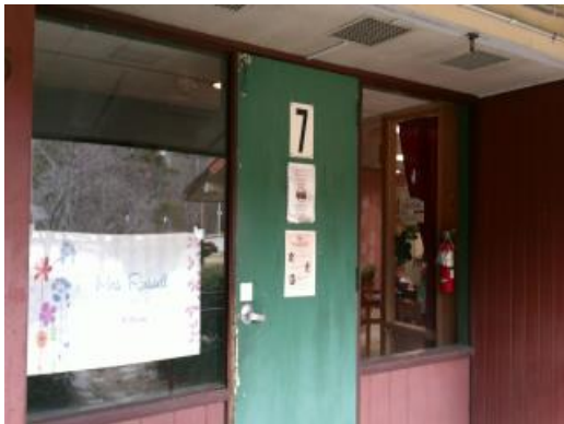
Faded Exterior Door
