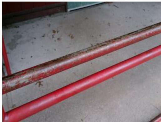
Typical Worn Handrail
