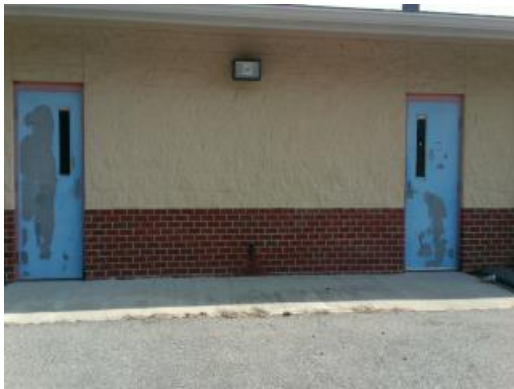
Typical Worn Metal Exterior Doors
