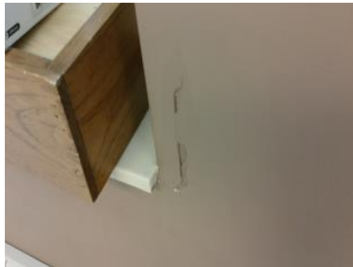
Damaged Gypsum Board Wall
