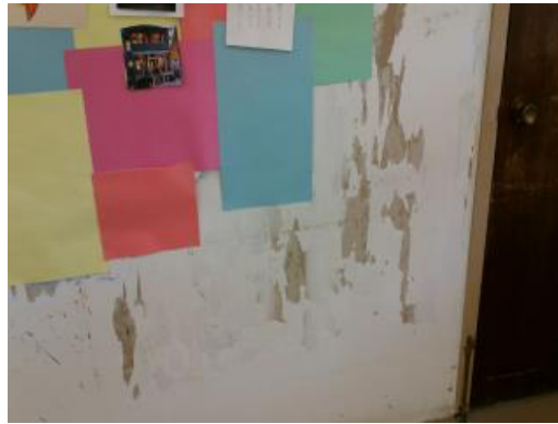
Main Building - Damaged Painted Classroom Wall
