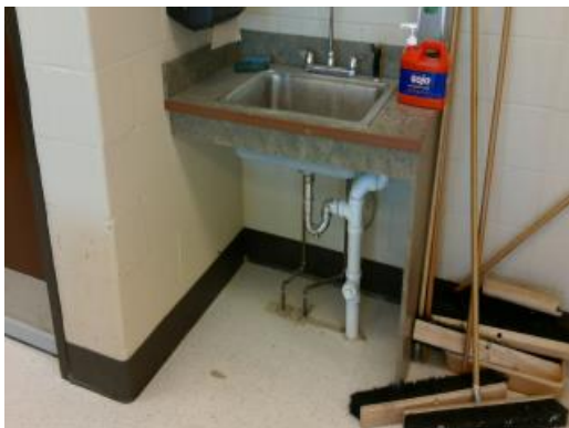
Pipe Missing Insulation
