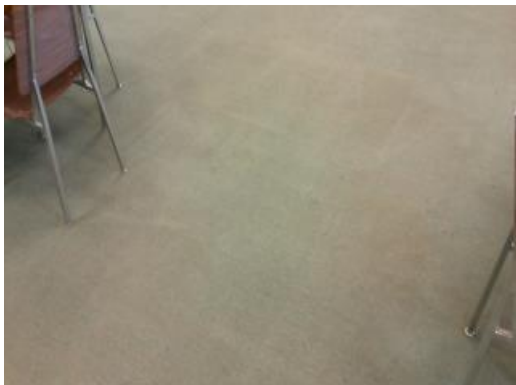
Main Building - Worn And Faded Carpet
