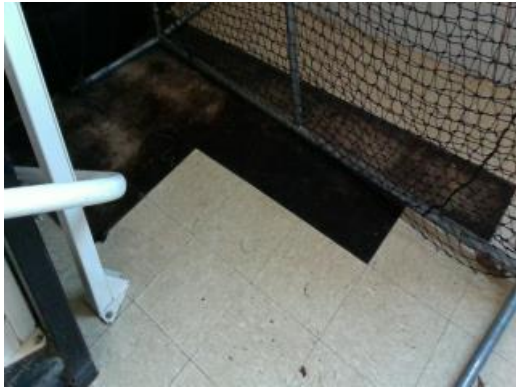
Main Building - Cracked And Missing VCT
