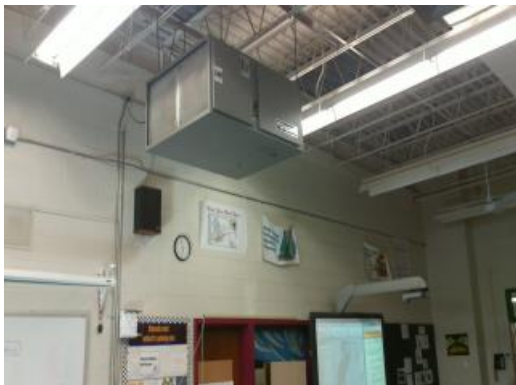
Main Building - Poorly Functioning Unit Heater
