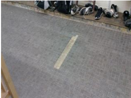
Main Building - Missing Ceramic Tiles
