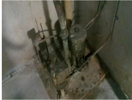
Main Building - Inoperable Sump Pump
