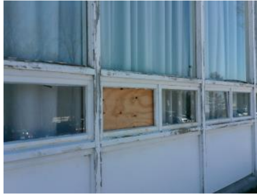
Main Building - Windows With Missing Pane
