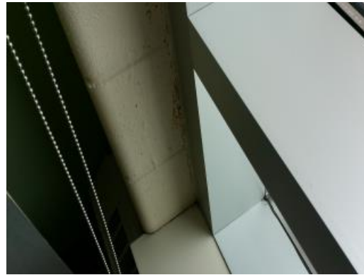
Failed Sealant Allowing Leaks
