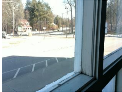
Main Building - Cracking Wood Framed Window
