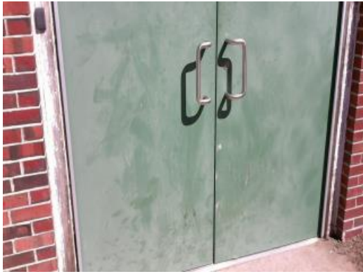
Main Building - Faded Metal Exterior Doors
