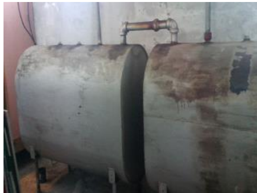
Fuel Oil Storage Tanks
