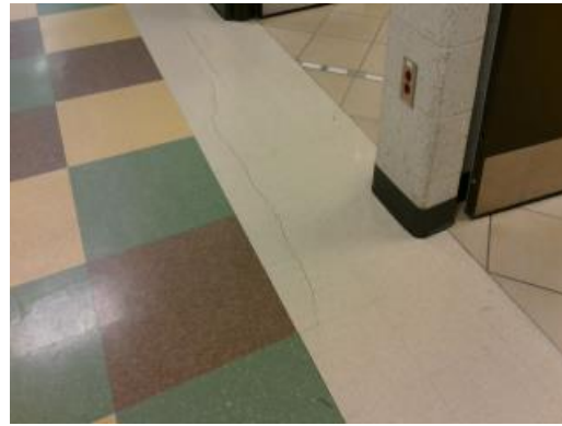
Cracked VCT Floor
