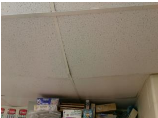
Bent Ceiling Grid
