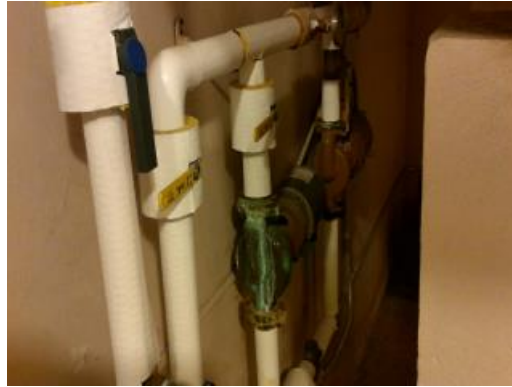
Main Building - Abandoned Circulators
