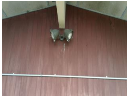
Building Mounted Light
