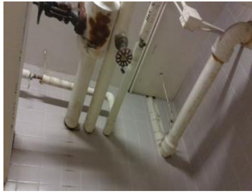
Main Building - Corrosion On Water Piping
