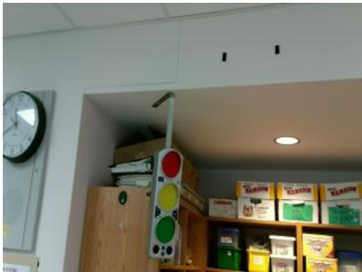
Cracks In Painted Walls
