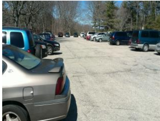
Site - Cracked And Worn Asphalt Parking Lot
