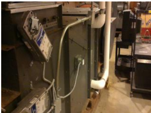
Main Building - Original AHU
