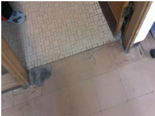
Typical Worn VCT
