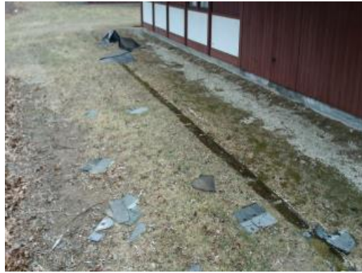
Displaced Roof Shingles
