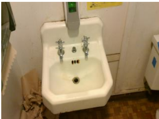
Typical Lavatory Fixture
