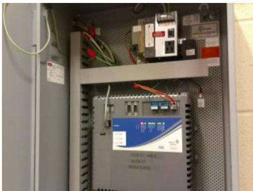
DDC Control Panel
