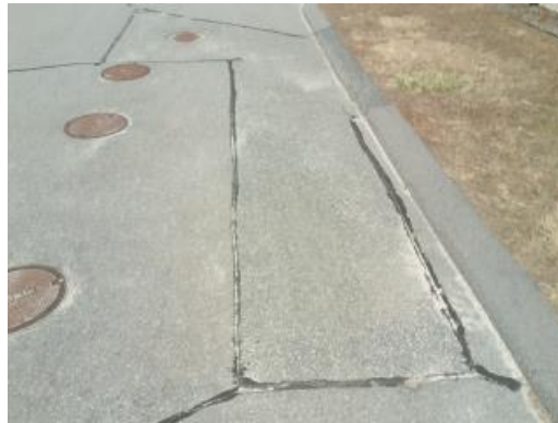
Damaged Play Area Asphalt
