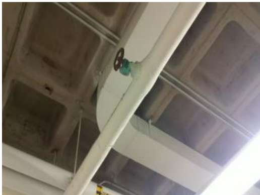
Main Building - Heating Hot Water Piping
