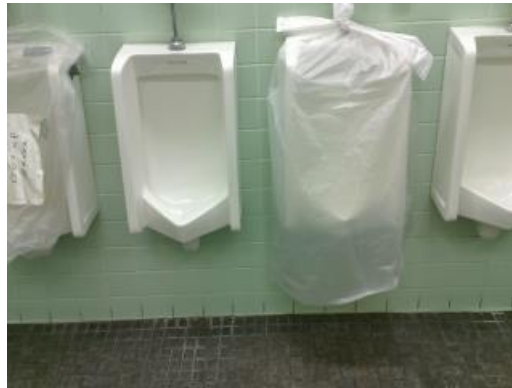
Main Building - Urinals Out Of Service
