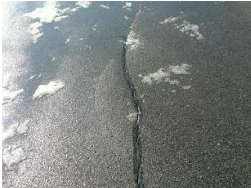
Cracking At Asphalt Joint
