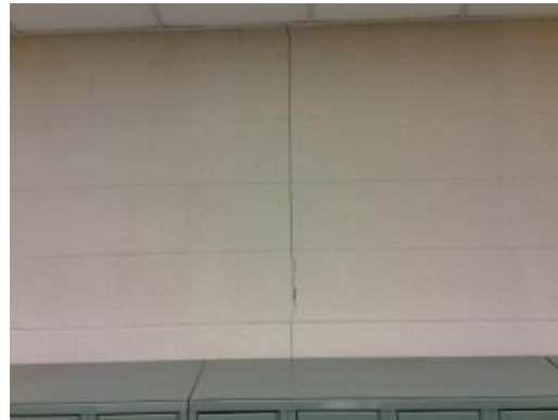
Cracked CMU Wall
