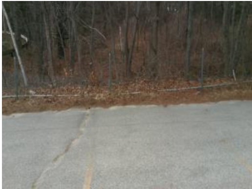
Fence Falling Down
