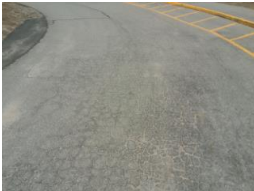
Cracking Asphalt Paving
