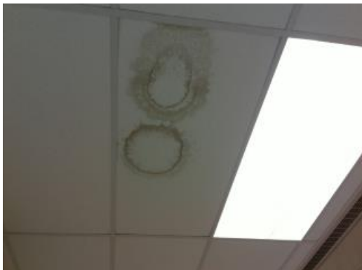
Stained Ceiling Tile
