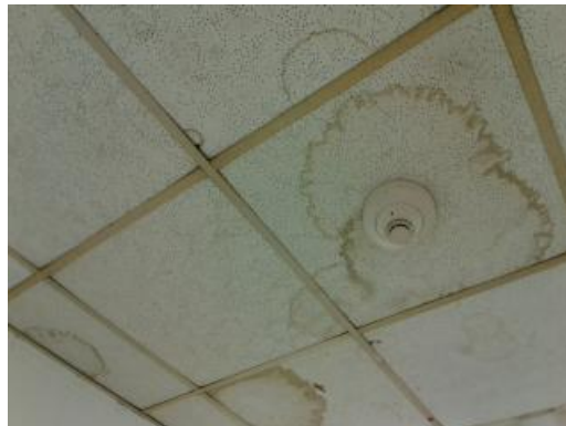
Main Building - Stained Ceiling Grid And Tiles
