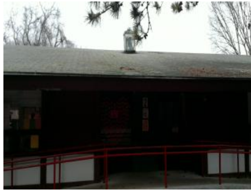
Shingles Missing From Building 2 Roof
