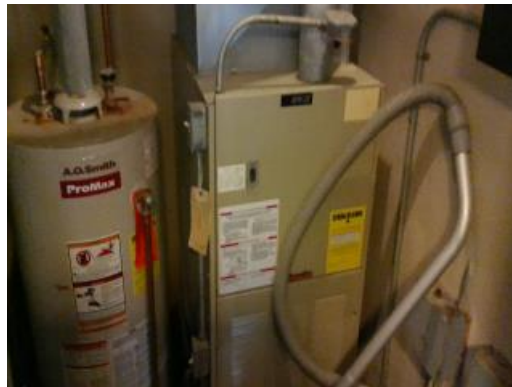
Furnace And Water Heater
