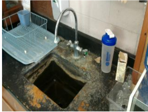
Main Building - Corroded Classroom Sink
