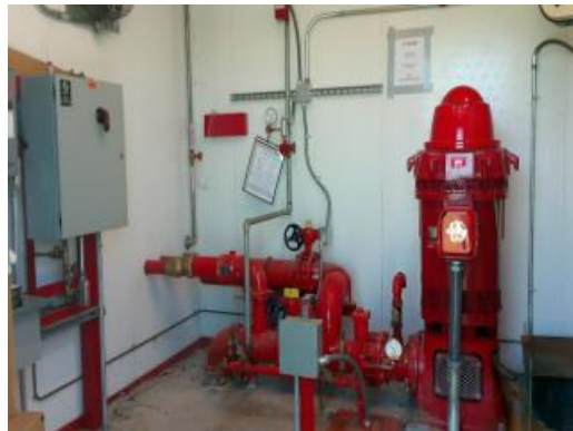
Fire Pump House - Interior
