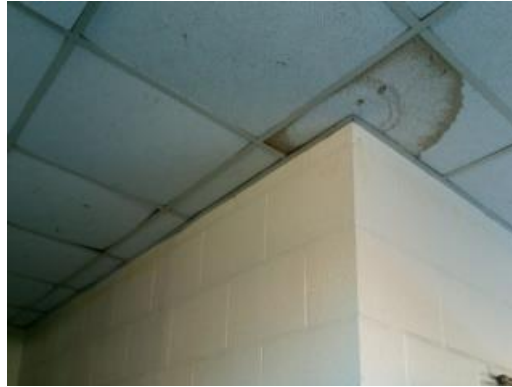
Main Building - Stained Ceiling Tiles
