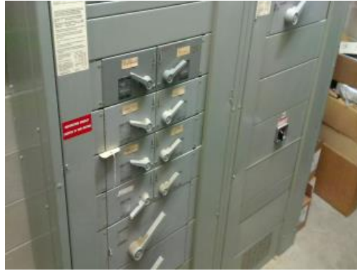
Main Distribution Panel
