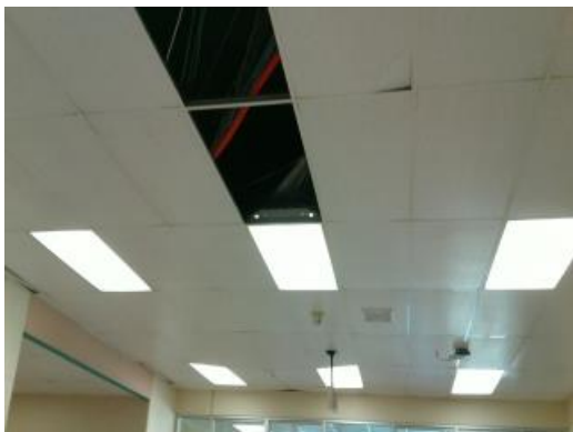
Missing Or Stained Ceiling Tiles
